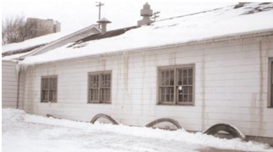
Extractive bleeding resulting from ice dams ▼
